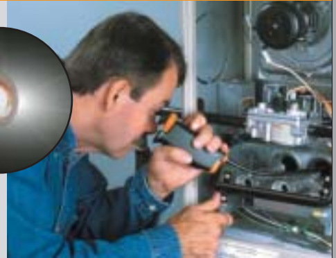
Inspecting a hard to reach point in a heating system
