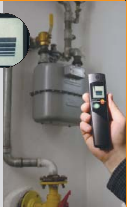
Audible warning about dangerous gas concentrations e.g. at gas pipe connections
