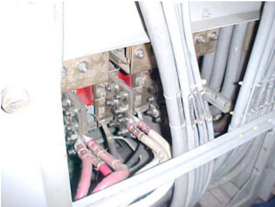
Figure 2. Switchgear test points
