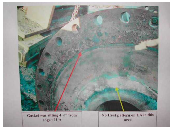
Figure 11. Flange gasket showing no burn marks
