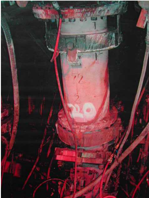
Figure 4. Blast furnace gimbal expansion joint
