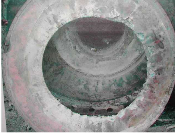
Figure 9. Partially destroyed upper assembly flange gasket
