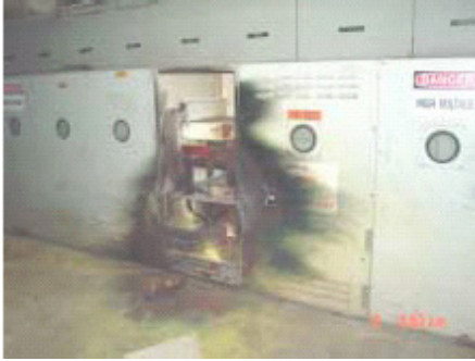
Figure 4. 4kV starter cell
