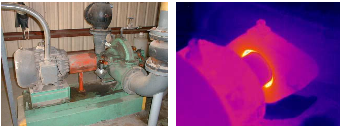
Figure 6. Visual and thermal images of a cooling water pump
